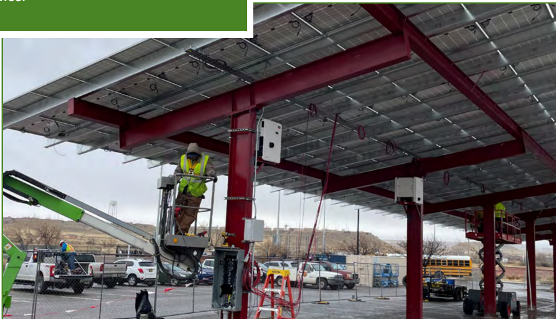
Tohatchi School solar canopy. Tohatchi, NM. Courtesy of Yearout Energy.
